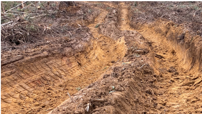
Example of an extraction track with machine rutting and no drainage.
